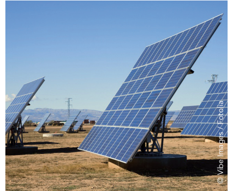
Control Unit / Solar
